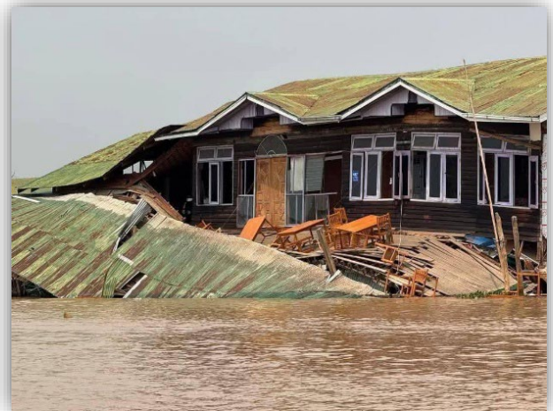
Inle Lake - destroyed buildings
