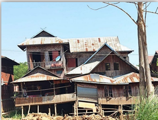
Damage houses in Sagaing
